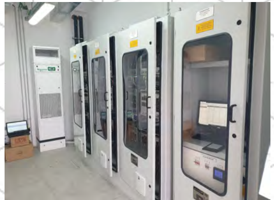
TR Units equipped with local and remote PC Monitoring & Control
