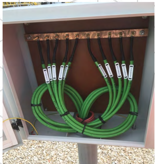
Junction Boxes and Test Stations
