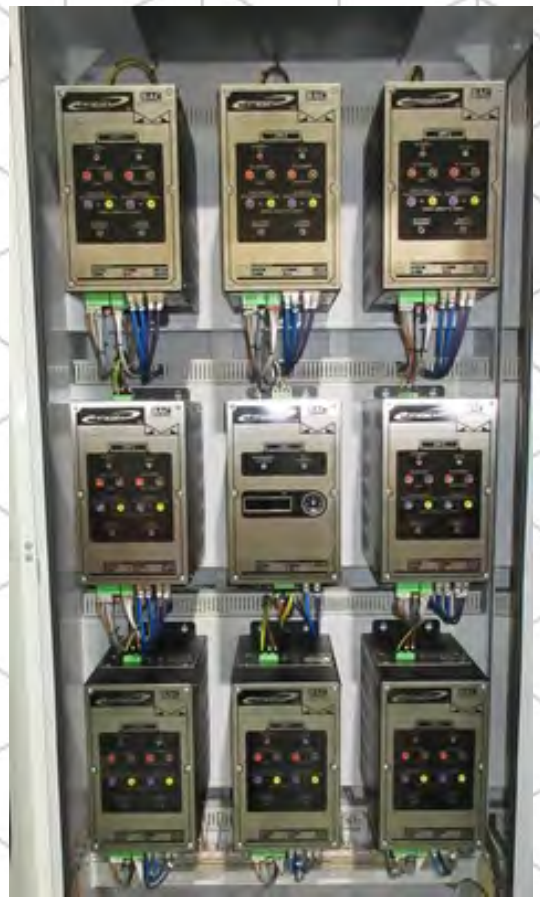
Thyristor Controlled Transformer Rectifiers
