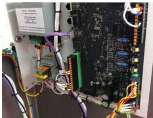
Infinity Control Board retrofitted to TR unit.
