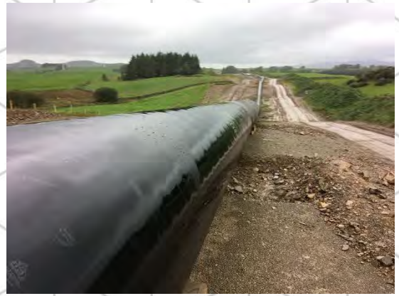
Pipelines new and old require Cathodic Protection and regular monitoring.
