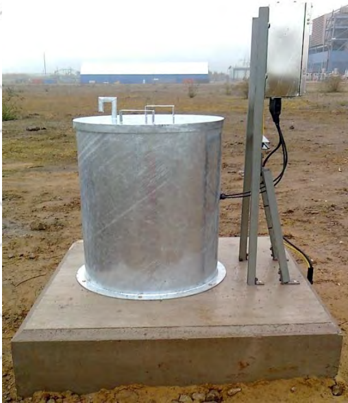
Deepwell grounded installation for pipeline ICCP system
